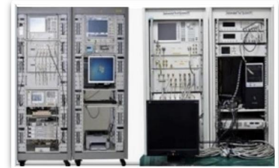
ATE ATS - Facility
